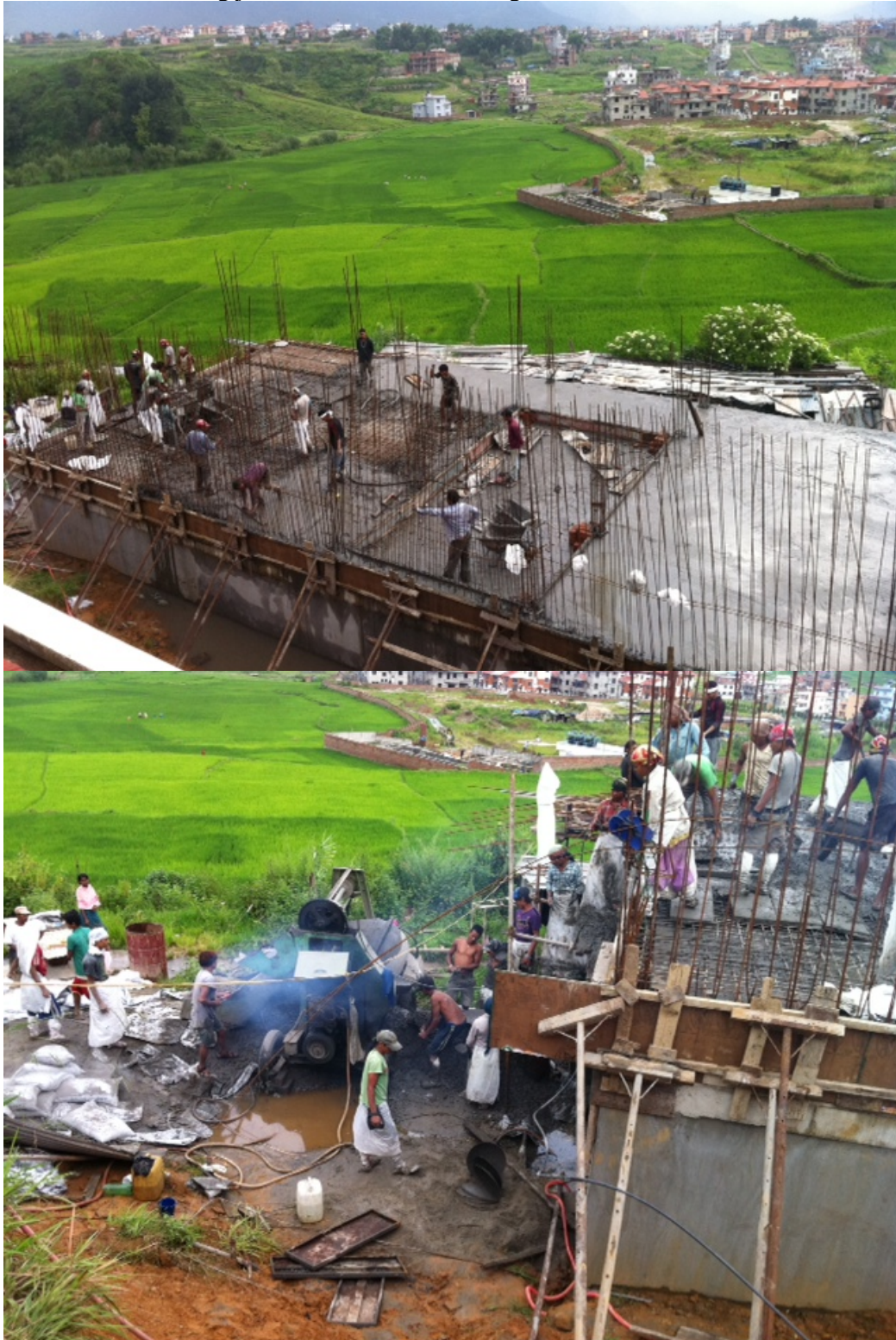
Casting the slab on the 1st floor of the dormitory building under construction!
