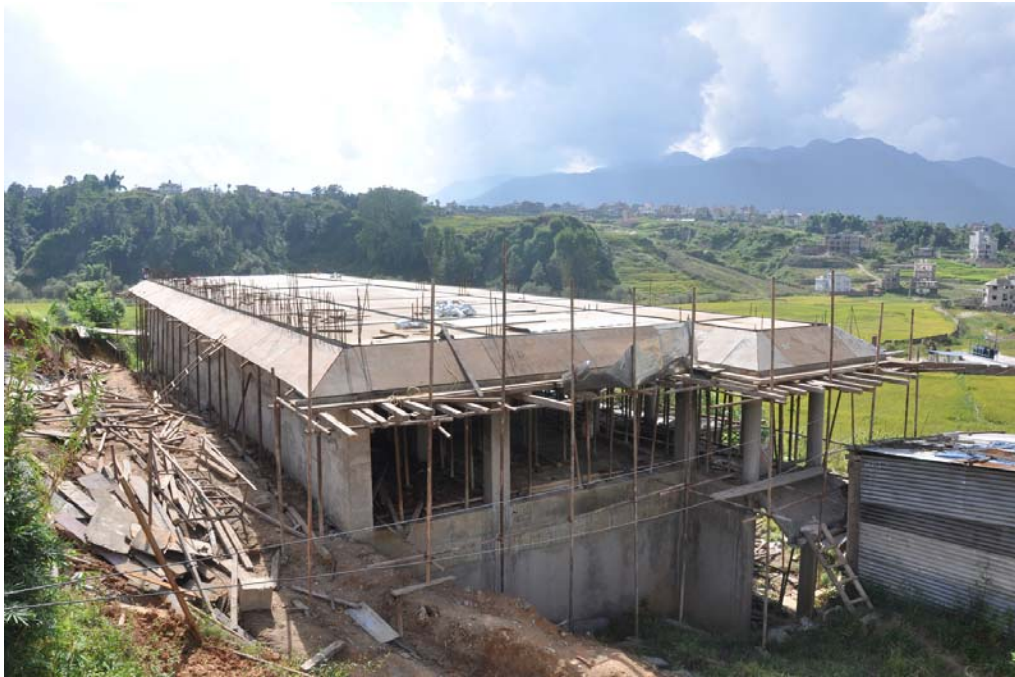
Just Ready for Casting after the Dasain Holidays – Photo Courtesy Sashank taken on 3 rd October
