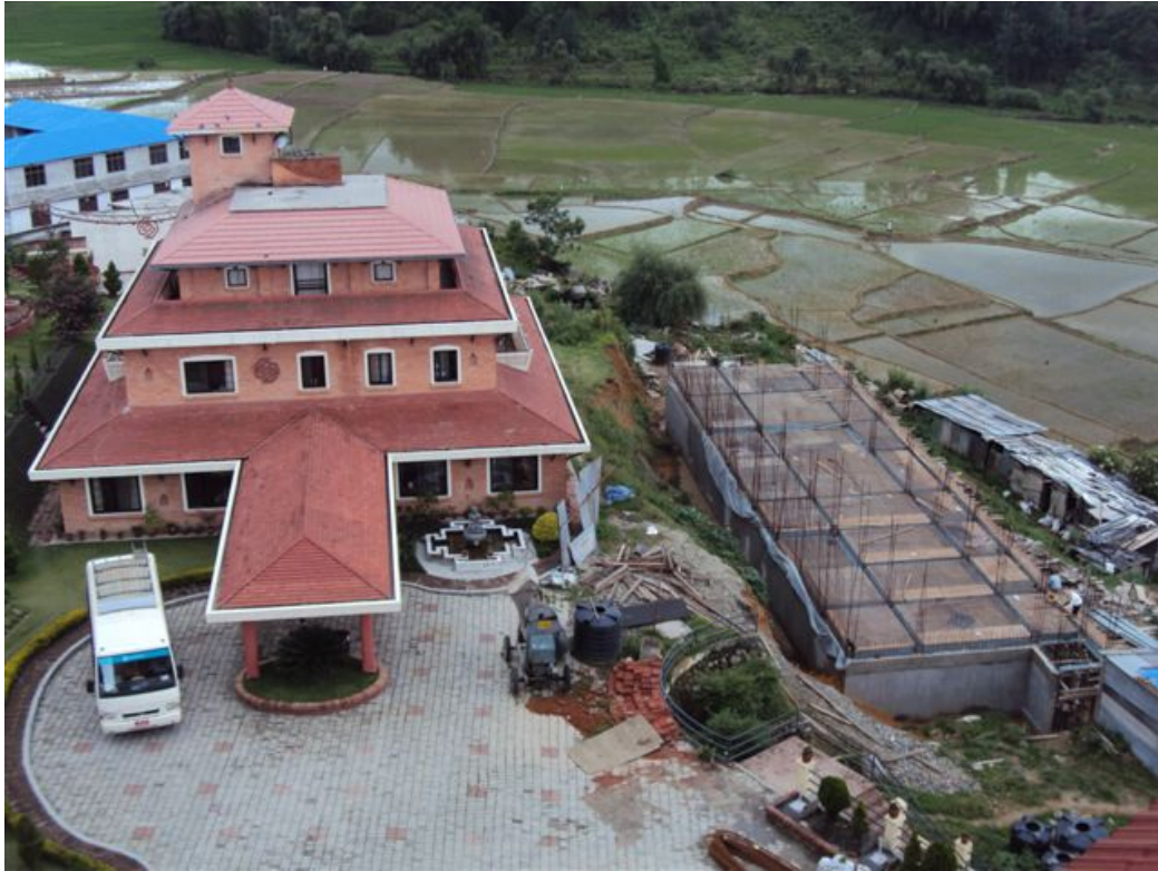
Shuttering work on the upcoming dormitory building (right) - the Tewa office on the left and the rice fields as backdrop!
