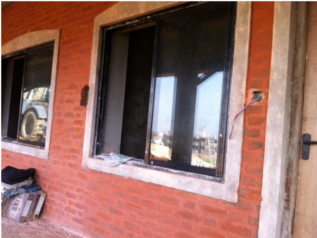
Details - Walls, Windows & Doors Completed. Many Details Remain! A leveling Bulldozer Reflected.
