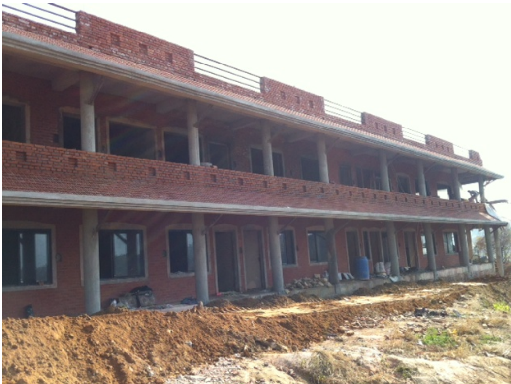
Dormitory Now – Please Note the Roof Top Terrace Wall, the Veranda Wall & Tiles on the Eaves!
