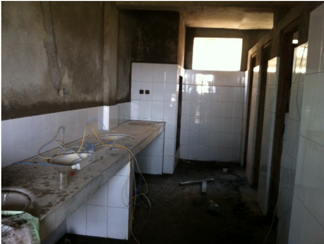
Common Bathroom – Fixtures, Floor, & Painting remains
