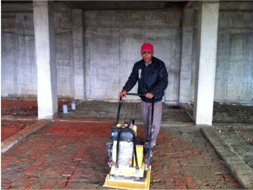
Prem, Long-time Tewa Site Supervisor is Compressing the Dormitory Ground Floor before PCC
